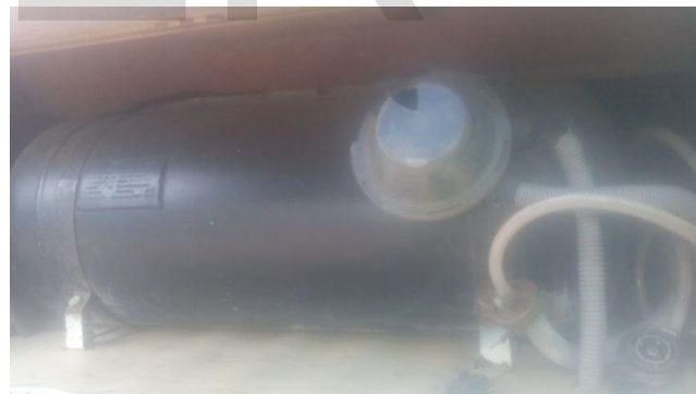
Fig. 2.2 Acetylene Storage Tank [3]
